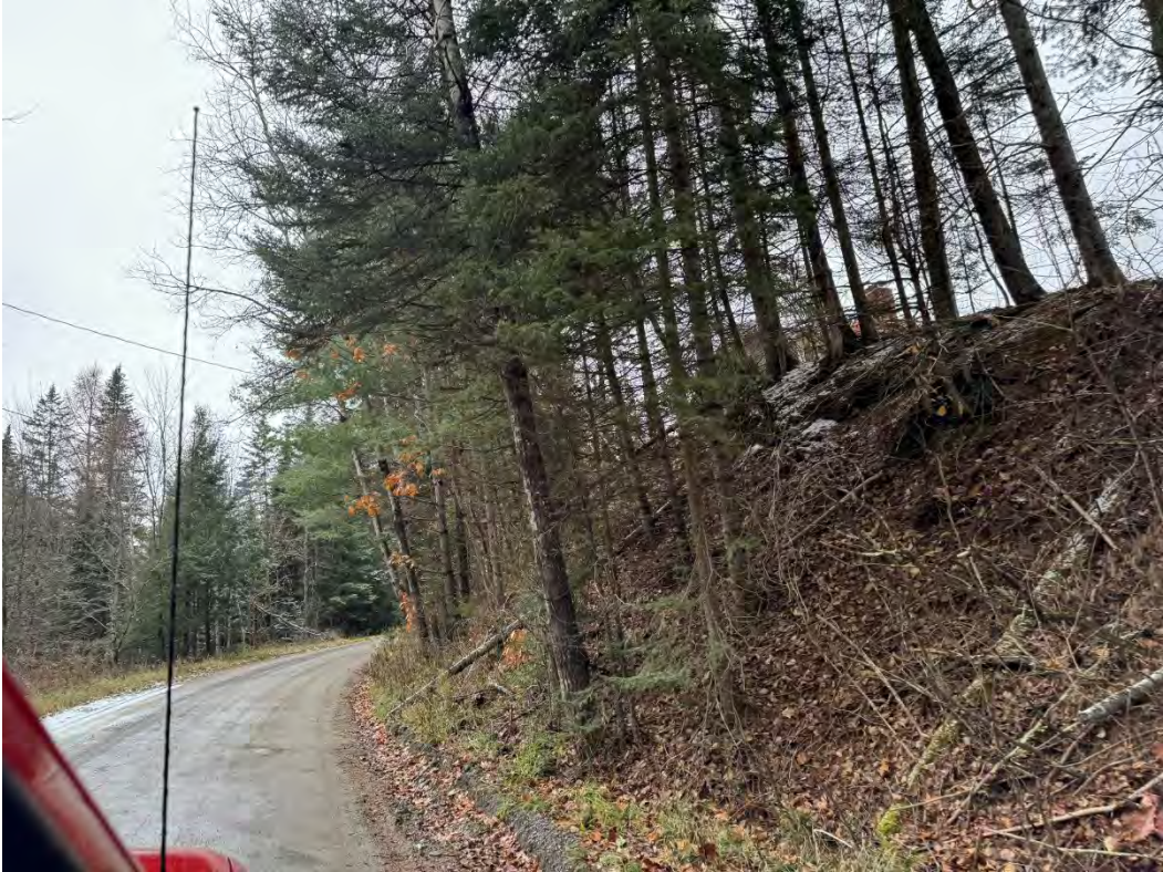
197568 before 2 – install stone line ditch on right side going uphill, tree removal
